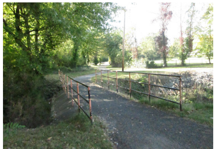
Greenway Bikeway: Existing bridge railings do not meet current standards and should be upgraded.
