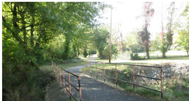
Greenway Bikeway: Existing bridge railings do not meet current standards and should be upgraded.
